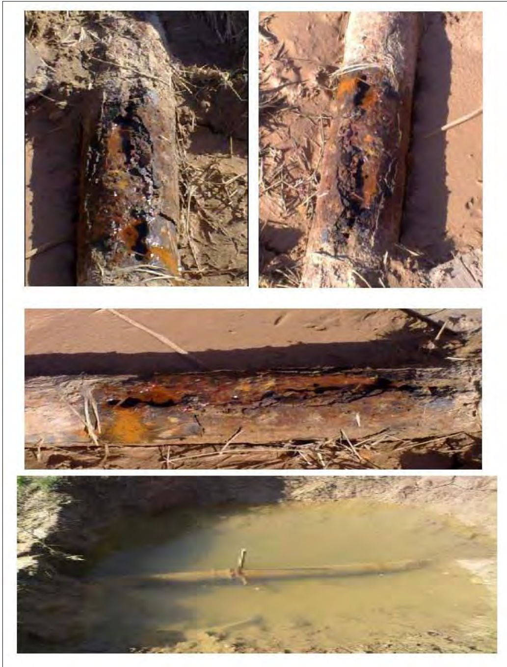
Corroded pipes of the drinking water network cannot be repaired due to the siege Foul water around corroded pipes gets into the drinking water network contaminating the water with infectious diseases
