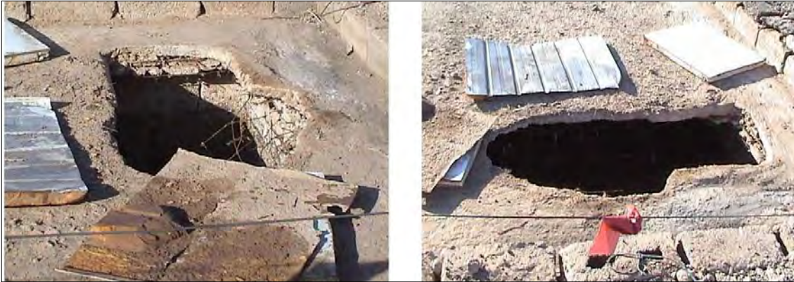
The concrete covers for black water tanks have collapsed posing a safety hazard to the residents
