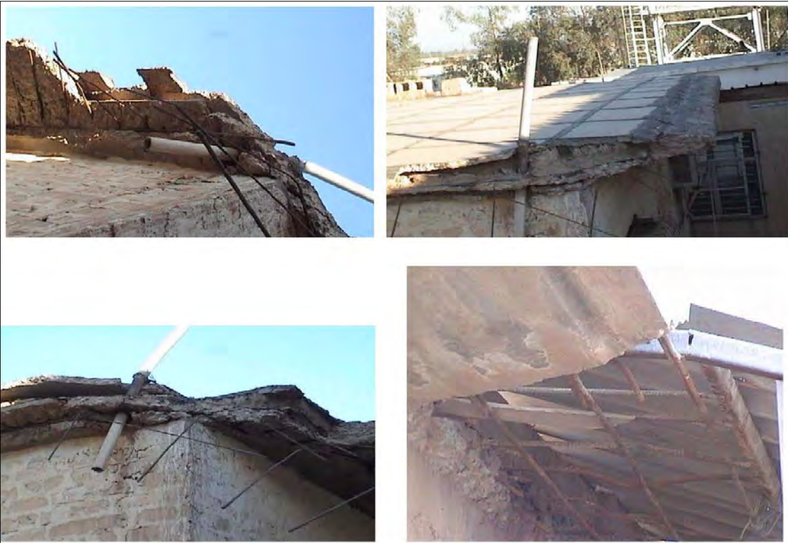
Risk of falling down of the ruined edges of ceilings
